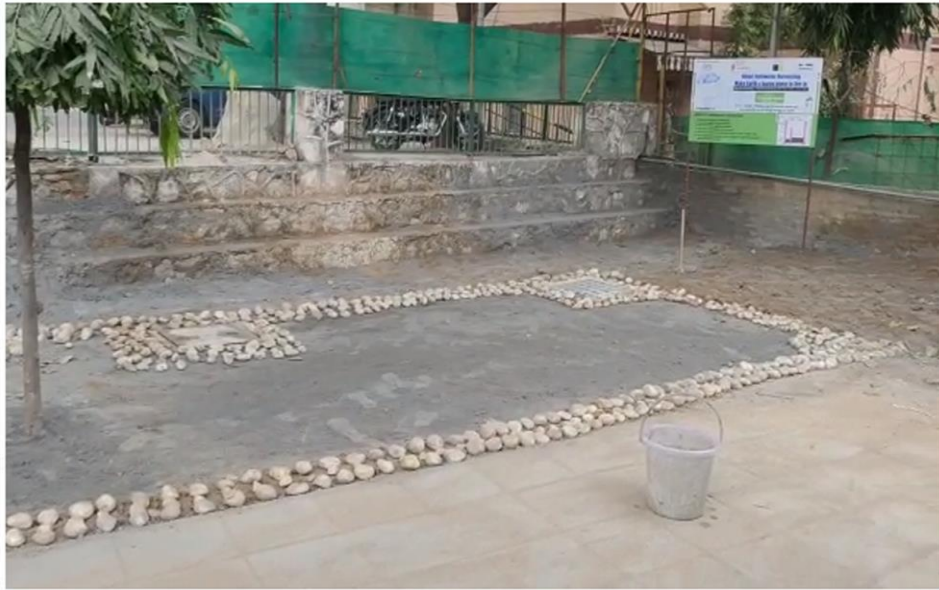
Rain Water Harvesting Structure – B-4 Vasant Kunj
